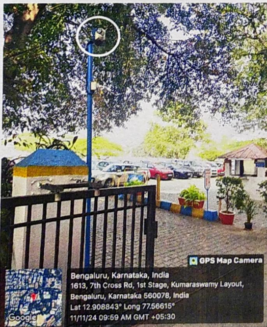
CCTV camera at the parking
